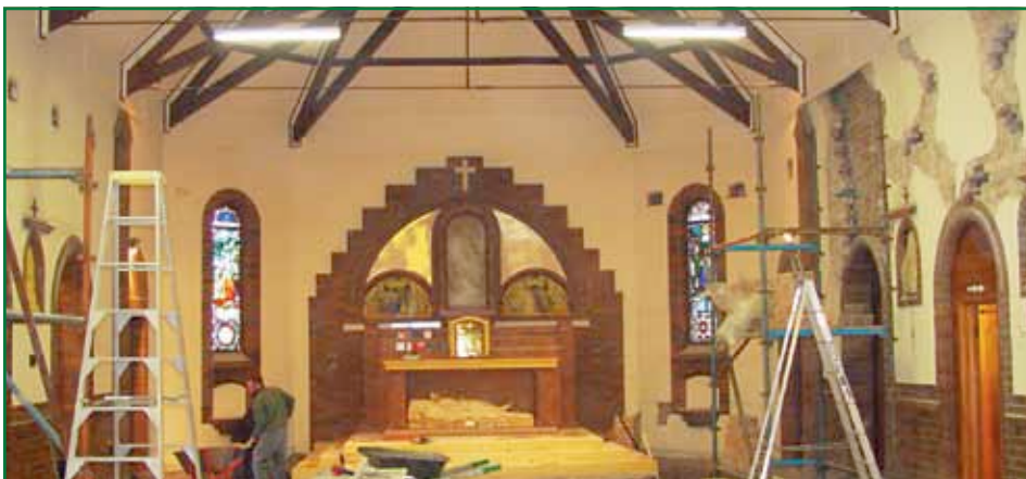
Bombala Church Repairs: St Mary's Bombala is cleared out for work to repair damage caused by an earth tremor
